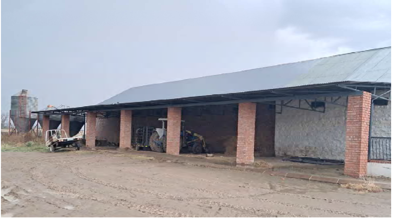
Figure 11: New addition to the existing barn (extended area) is clearly visible by the use of facebrick.
