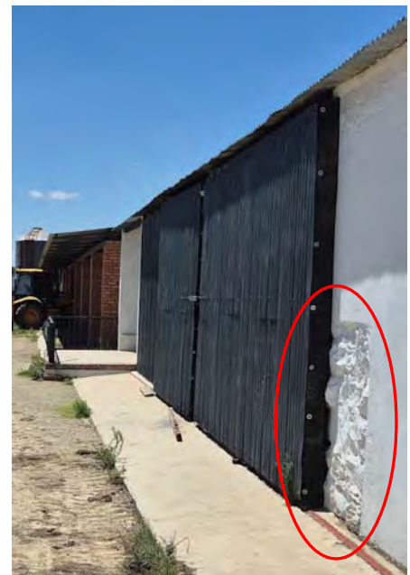
Figure 7: Section of historic barn that was not plastered reveals its original building material
