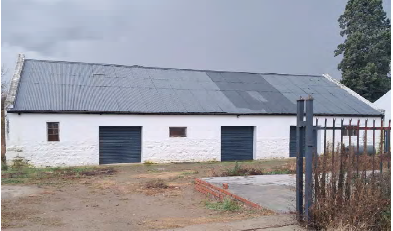
Figure 9: Alterations made by previous owner on the rear end of the homestead
